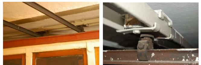
Fig. 14.: The double pole feeding rails with wooden insulator-holder (URM)
