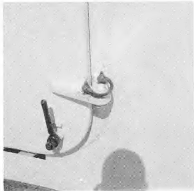
Figure 2. Ground Strap on Water Tight Door
