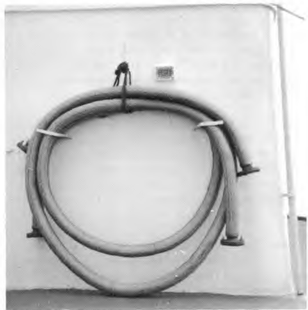
Figure 7. Flexible Vent Hose Stowed Topside was Relocated for Storage Inside.
