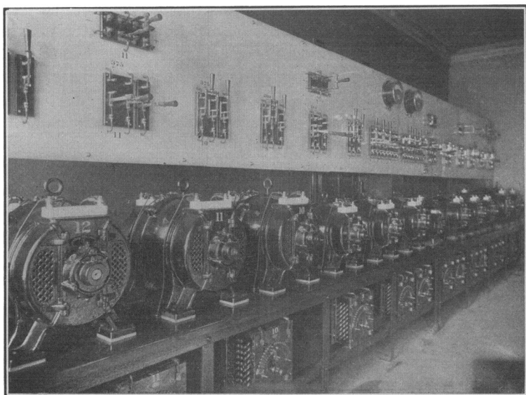
FIG. 2a.—Typical arrangement of motor dynamos in telegraph work
