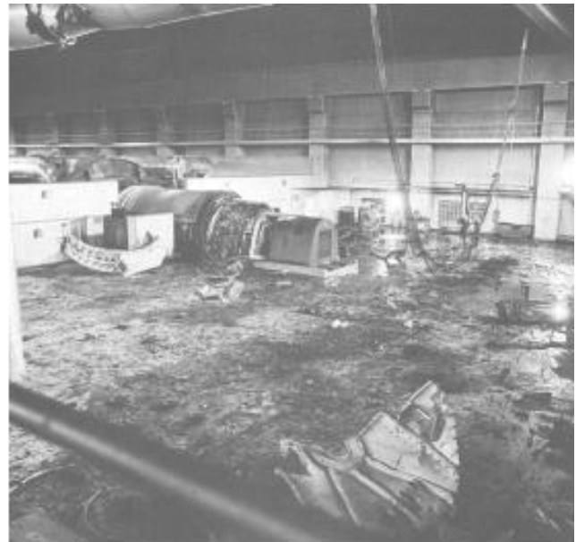
Figure 7. Barsebäck generator hall after retaining ring fracture in April 1979.
